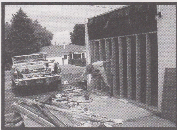
A new wall was put in where there was a garage door opening into the library's "back room." Independent contractor Steve Benson did the work.
